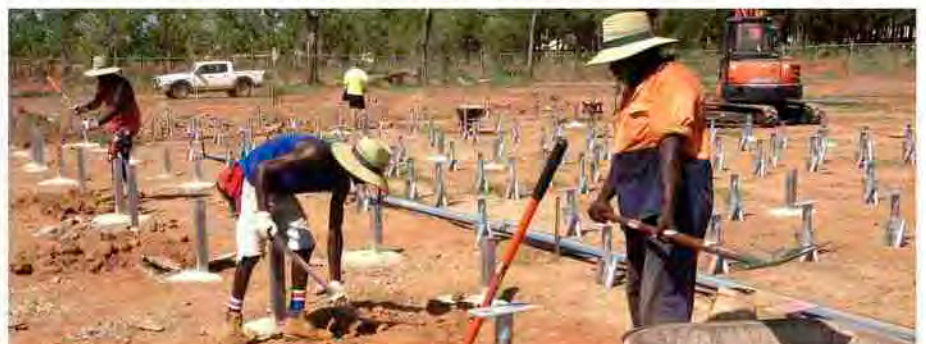
Greg Orsto, Ambrose Munkara and Harvey Darcy at work at new Shopping Centre construction site
